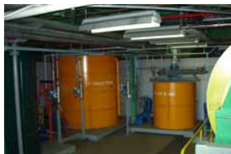
Painted and Operational
